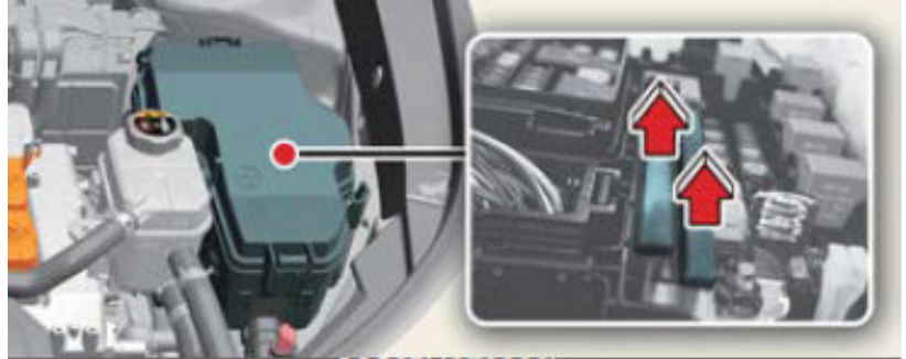
Engine room fuse box
